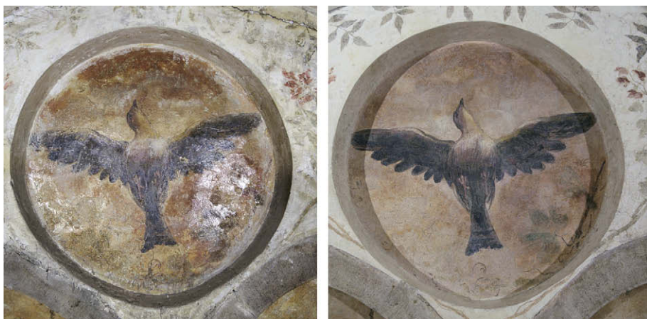
Fig. 2. Wall paintings in San Salvador church in Venice: pre- (left) and post-removal (right) of Paraloid B72.
