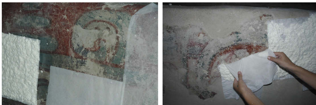
Fig. 7. Different steps of an in situ application of nanoparticles dispersions (credits by Alice Desprat).
