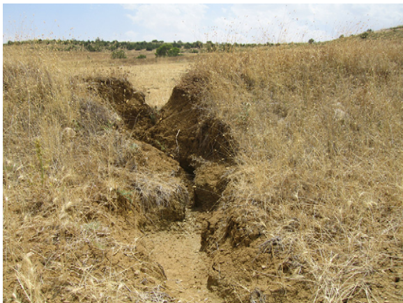
Fig. 6. Example of a breach on a contour bench at the El Gouazine catchment area.
