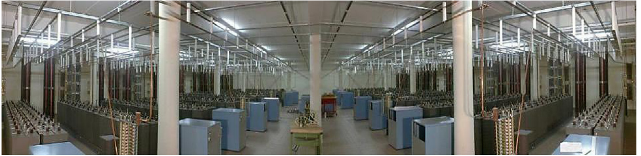
Fig. 2. Top: the basic circuit of a capacitor bank showing the main components: a dump resistor with a discharge switch, the storage capacitors protected by a fuse (fuse not shown, normally a large number of capacitors is in parallel and every capacitor is protected by a fuse), a crowbar diode and its resistor to create an exponentially decaying field and to limit the voltage reversal on the capacitors, a self-inductance to limit the current in the installation in case of a short, the high-voltage charger (normally a voltage limited current source), a switch (in nearly all cases a thyristor, except for single-turn coils) to connect the stored energy to the user coil, and finally the user coil that has an inductance and a history dependent resistance. Bottom: a fish-eye view of the 14 MJ capacitor bank as installed at the pulsed facility LNCMI-Toulouse (blue cabinets are the chargers, grey boxes are the capacitors and the cylindrical structures at the back are the protecting self-inductances). (For interpretation of the references to colour in this figure legend, the reader is referred to the web version of this article.)
