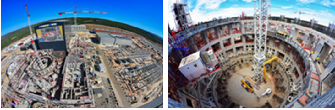
Fig. 2. (a) Little free space remains on the 42 hectares of the ITER platform. Sandwiched between the cooling tower zone and concrete batching plant at the northern end (far left) and the electrical switchyard to the south (far right) are the work areas for the Tokamak Complex (centre crane), the cryoplat (middle right, all grey) and the buildings for magnet power conversion (twin structures, right). Any free space is used for storage. At the top of the image, manufacturing is underway in on-site facilities for the cryostat and four of the machine's six poloidal field coils, too large to be transported by road. (b) The ITER tokamak will be assembled in this "well" at the centre of the Tokamak Complex building. The large openings in the walls of the "bioshield" – the thick steel and concrete structure that surrounds the machine – are "penetrations" that will allow system equipment such as magnet feeders, remote handling, heating and diagnostics to reach the machine.
