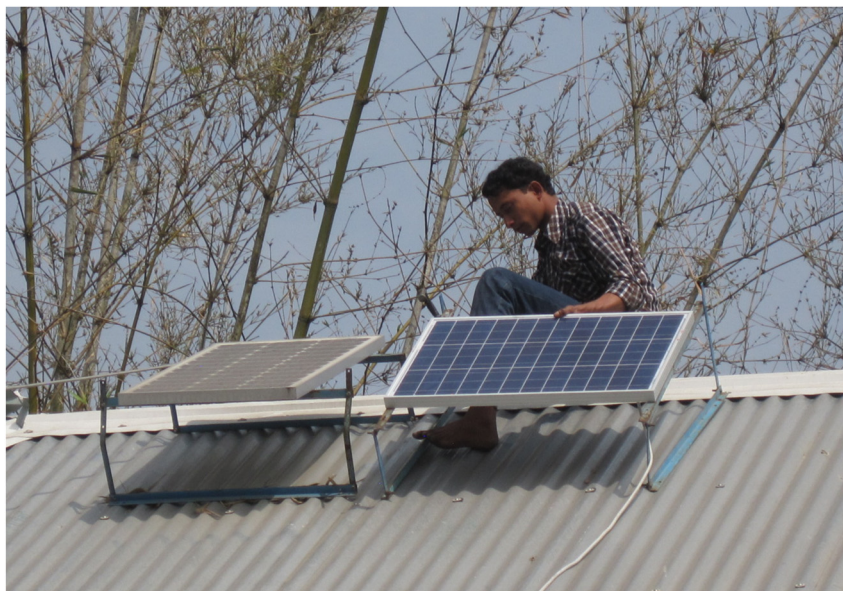
Fig. 3c. In Bangladesh, installing a solar module for a solar home system on a roof (photo: A. Jacobson).
