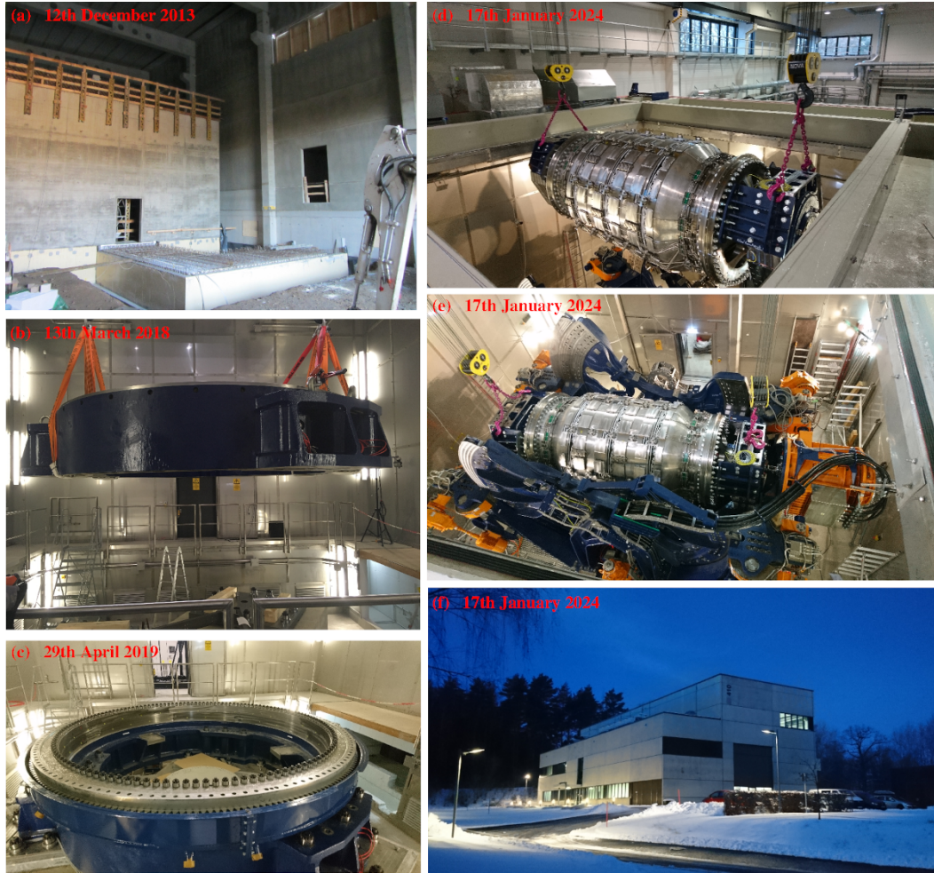
Figure 9. Some impressions from the construction, with relevant dates indicated. (a) Shell construction of the containment and the air duct (for cooling). (b) Insertion of the underframe. (c) Slewing bearing mounted on the underframe. (d) and (e) Insertion of the vessel into the frame. (f) The DRESHDYN building.
